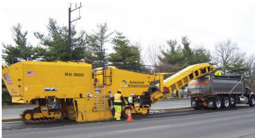
On March 4, Maryland awarded a $2.1-million road resurfacing and improvement project along New Hampshire Avenue in Montgomery County to American Infrastructure. (Photo courtesy American Infrastructure)
