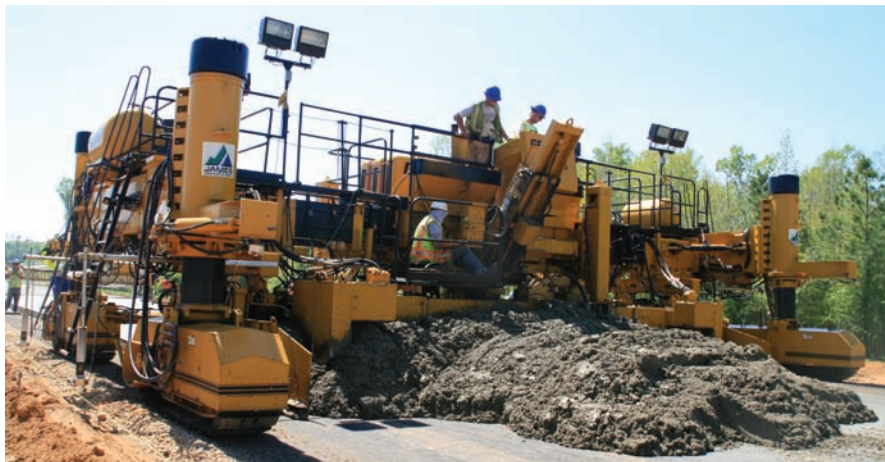
The $298 million in stimulus funds that will go to the Louisiana Dept. of Transportation and Development will create a statewide ripple effect. James Construction Group of Baton Rouge, La., paves two new lanes on US 167 in north Louisiana. (Photo by Sam Barnes)
